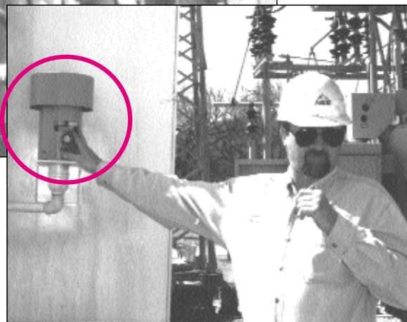
James Mitchell, NES supervisor--underground and substation, specifies Des-Case breather models CS-6 for NES oil tankers.
